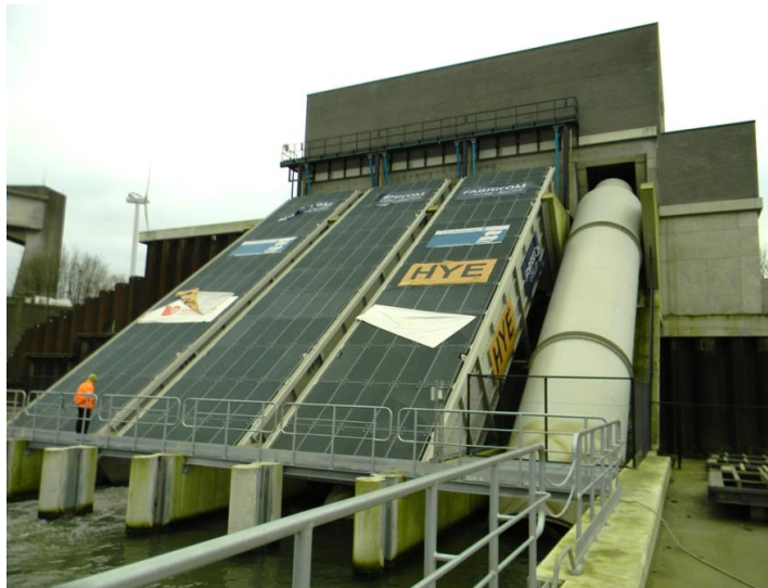
Fig. 11.1 The hydropower station of Ham (Belgium), equipped with three Archimedes hydrodynamic screws (on the left; the cover does not turn with the screw and is fixed; the screws can pump water and generate power as turbine), and one true Archimedean screw (on the right, the cover is fixed to the screw and turns with it; this screw can only pump water)
