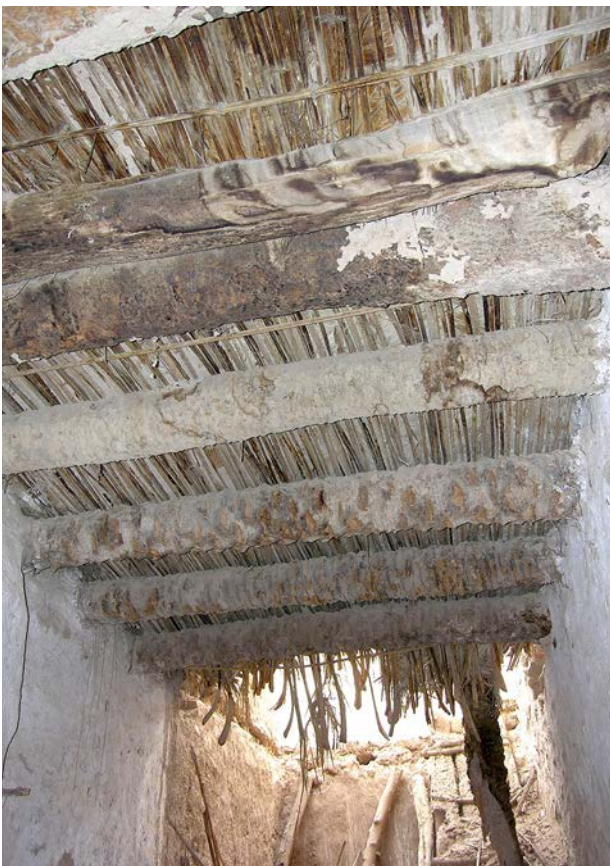
Fig. 15. The roofing in traditional 19th–20th century houses in the Old Town of al-'Ulâ (Z.T. Fiema).
