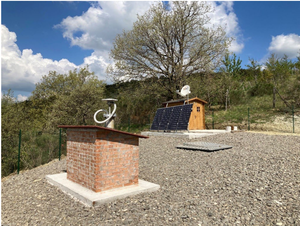
Figure 5. TSM2 observatory site: a single site hosting strain- and seismo-meters within a 160 m deep borehole, roundtrip fibre optic cable and pore pressure gouge within a pipe installed within the same hole. At the well head, covered by the small brick cottage (on the left), is visible the GNSS antenna, while in the centre of the picture there is the aluminium cover to protect the sensor pocket installed on the surface. On the right, the wood house hosting the acquisition and satellite transmission system with Meteo antennas on the roof. The power system composed by a set of solar panels are placed in the front of the house.
