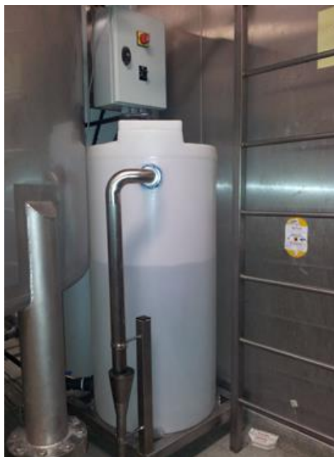
Figure 2. RO Wastewater Tank
