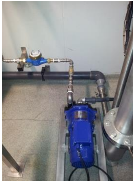
Figure 3. Wastewater Recovery Pump and Counter
