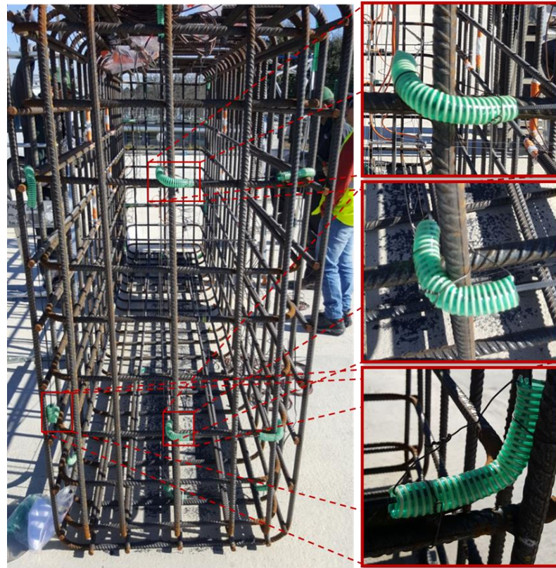
Figure 11. Instrumentation of block KB with embedded DOFS and details of cable bends around the stirrup (pictures on the right side).
