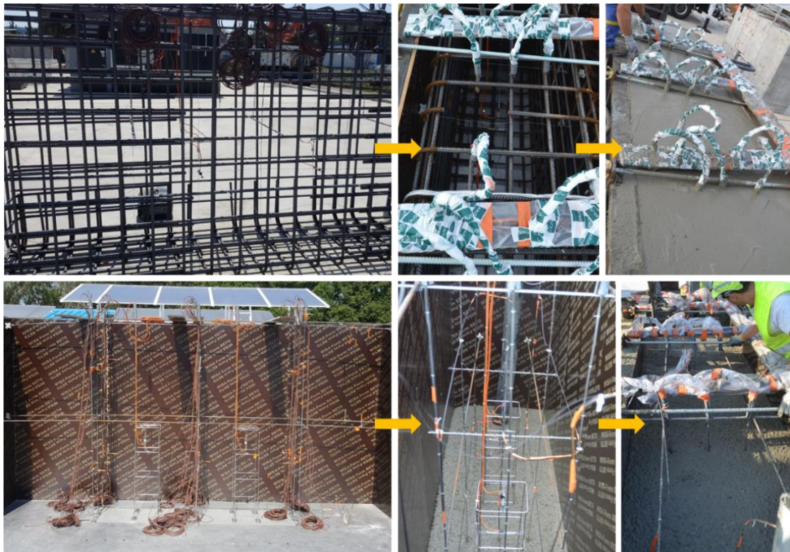
Figure 4. Construction steps of the two types of ODOBA blocks: RC blocks (top pictures) and NRC blocks (bottom pictures).
