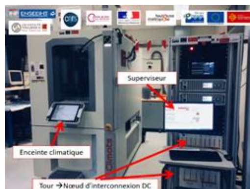
Figure 23 : Battery test bench
