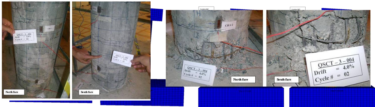
Figure 8: Failures observed in the experimental test a) Tensile cracking, b) Compressive crushing of concrete and rebar yielding
