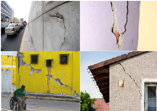
Fig. 12. Samples of images with cracks taken from the Internet.
