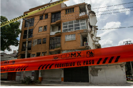
Fig. 1. Damaged building during an earthquake in Mexico in 2017.
