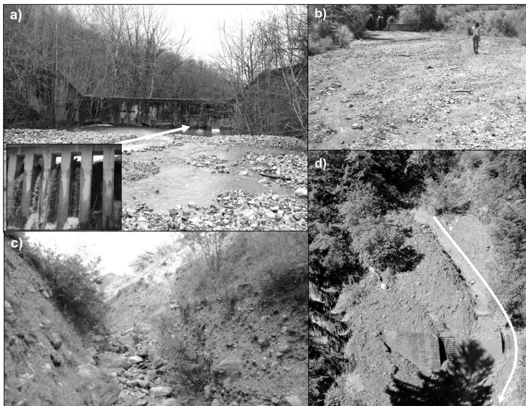
Figure 13.5: Illustration of main malfunctions identified for sediment traps: a) decrease in the retention capacity due to wood logs frequent clogging in the Lavanchon torrent (Saint-Paul-de-Varces, France); b) no more too costly dredging in the Clavaux torrent (Barcelonnette, France); c) location too far from elements-at-risk upstream and stopping of materials and filling for frequent floods resulting in downstream bed incision in the Manival torrent, (Saint-Ismier, France); d) bypass of the open check dam by right side in the Castelvieil ravine (Luchon, France)
