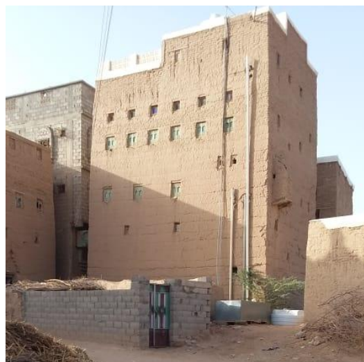
Water drainage system with pipes that requires a special attention to the wastewater drainage on the ground – ©CRAterre
