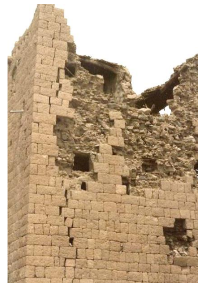
Destruction after the earthquake of Dhamar in 1982, no tie/through-stone in the wall – source Sjoerd Nienhuys 1984
