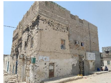
Some combination between traditional and industrial material can lead to severe structural disorder, Shabwa Gov., Rodhom dist. 2022 – ©YFCA
