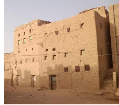
No foundation in flash flood prone area can be disastrous, Shabwa Gov., Almarkha alsofla Dist. 2022 – ©YFCA
