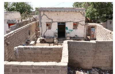
Unavailable skilled masons and high cost of cement and steel bars impact the quality of concrete housing, AlHudaidah Gov., AlKhokha Dist. 2020 – ©YFCA
