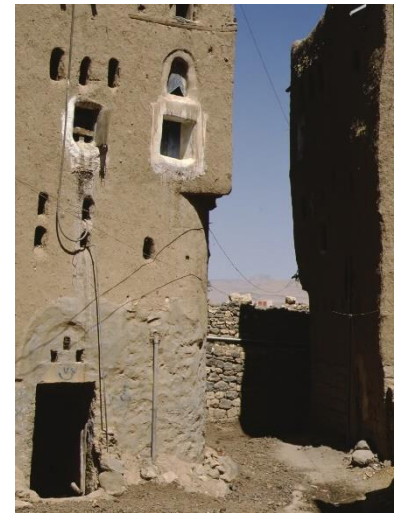
Cantilever in a building angle that widens street passage, Amran Gov. – ©CRAterre
