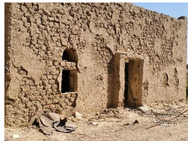
Earth brick, damaged earth plaster, Al-Jawf Gov., Almttoon district, 2021 – ©YFCA
