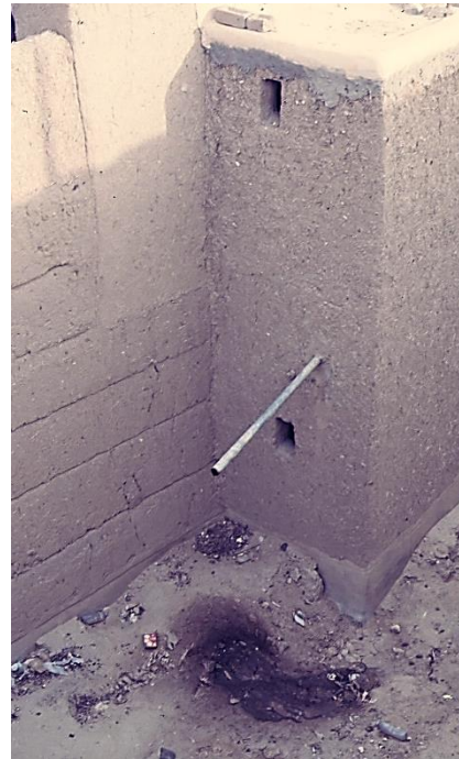
Traditional water drainage system that can have severe impact on the earth building footings when the running water system is introduced that increases water consumption – ©CRAterre
