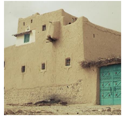
Waste drainage that may impact the foundation – ©CRAterre
