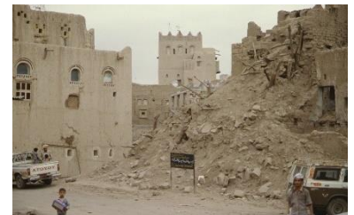
Lack of regular maintenance of earth building can lead to collapse, Amran Gov. – ©CRAterre
