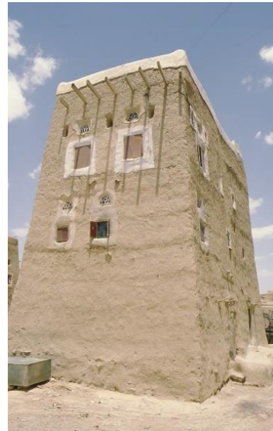
Well maintained cob wall house with lime plaster to protect the walls capping – ©CRATerre
