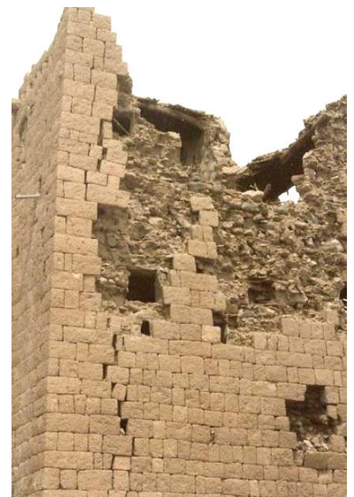
Destruction after the earthquake of Dhamar in 1982, no tie/through-stone in the wall – source Sjoerd Nienhuys 1984
