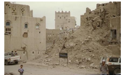
Lack of regular maintenance of earth building can lead to collapse, Amran Gov. – ©CRAterre
