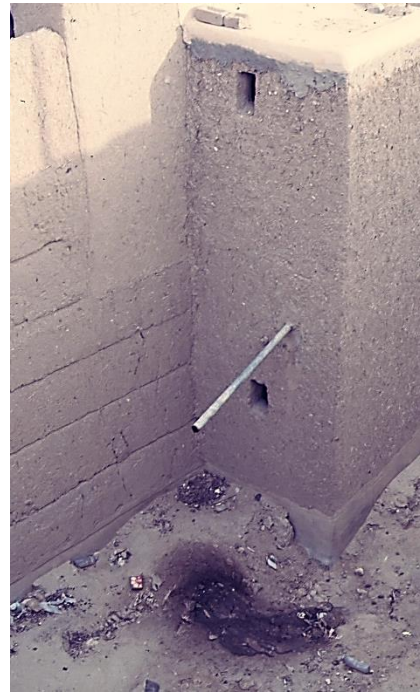
Traditional water drainage system that can have severe impact on the earth building footings when the running water system is introduced that increases water consumption – ©CRAtterre
