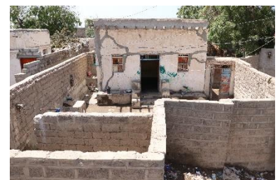
Unavailable skilled masons and high cost of cement and steel bars impact the quality of concrete housing, AlHudaidah Gov., AlKhokha Dist. 2020 – ©YFCA
