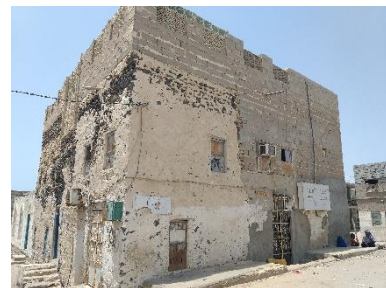
Some combination between traditional and industrial material can lead to severe structural disorder, Shabwa Gov., Rodhom dist. 2022 – ©YFCA
