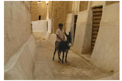
Protection of the base of the wall with wear mass of earth – ©Max Cortesi
