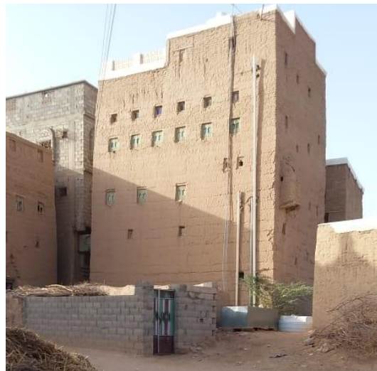
Water drainage system with pipes that requires a special attention to the wastewater drainage on the ground – ©CRAtterre
