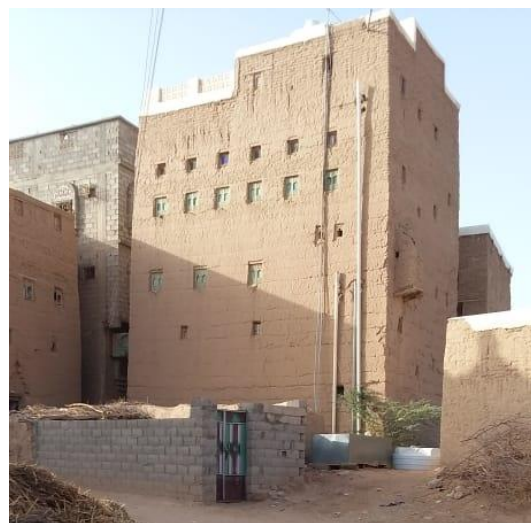
Water drainage system with pipes that requires a special attention to the wastewater drainage on the ground – ©CRAterre
