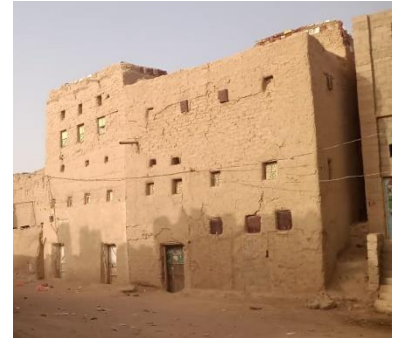
No foundation in flash flood prone area can be disastrous, Shabwa Gov., Almarkha alsofla Dist. 2022 – ©YFCA
