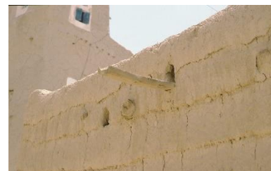
Good top roof drainage system made of wood, rain water is evacuated far from the façade – ©CRATERre
