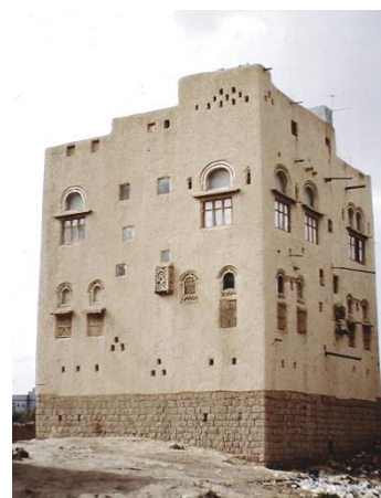
A base in stone masonry protect the building against flash flood – ©CRATerre
