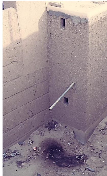
Traditional water drainage system that can have severe impact on the earth building footings when the running water system is introduced that increases water consumption – ©CRAterre
