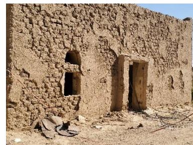
Earth brick, damaged earth plaster, Al-Jawf Gov., Almtoon district, 2021 – ©YFCA
