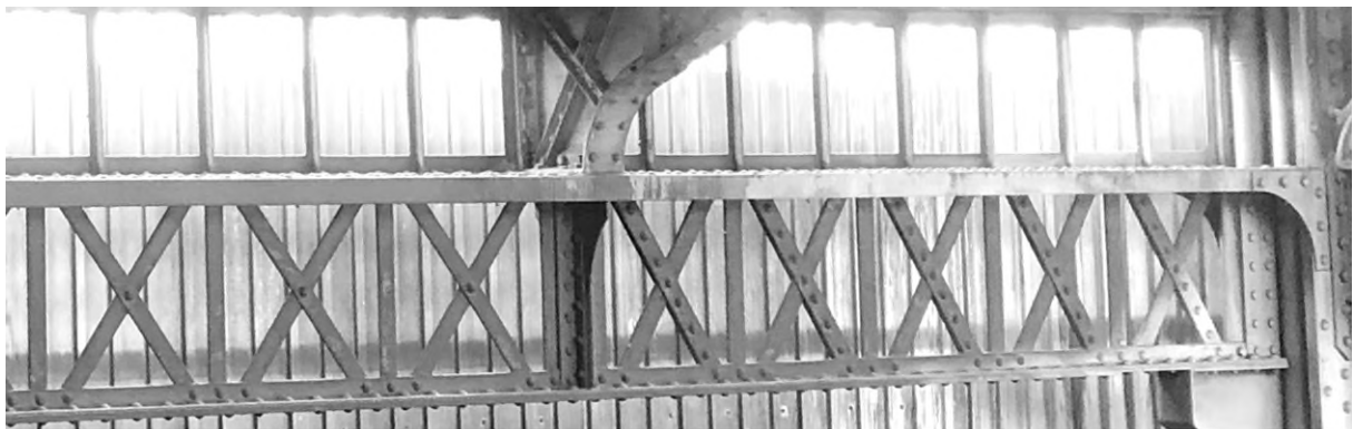
Figure 5: Trussed lower purlin at the Gare de Lyon-Perrache (halle St-Etienne, built in 1885). Photo: H. Franz.
