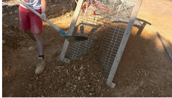
752 753 Figure A.1: Manual dry sieving prior to an earth-hemp formwork. On this building site, the sieve mesh size 754 was close to 1 cm, illustrating the variability of sieving objectives on field. Liquid state sieving is also a 755 common practice.
