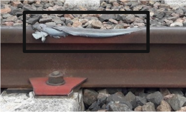
Fig. 1. Rail damage due to wheel-slip event in France; the squared area is the result of damage to the rails caused by train wheels.
