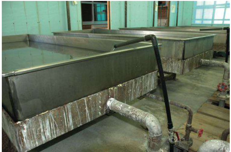
PHOTO 16 Injection of raw seawater through the seawater injection pipe.
