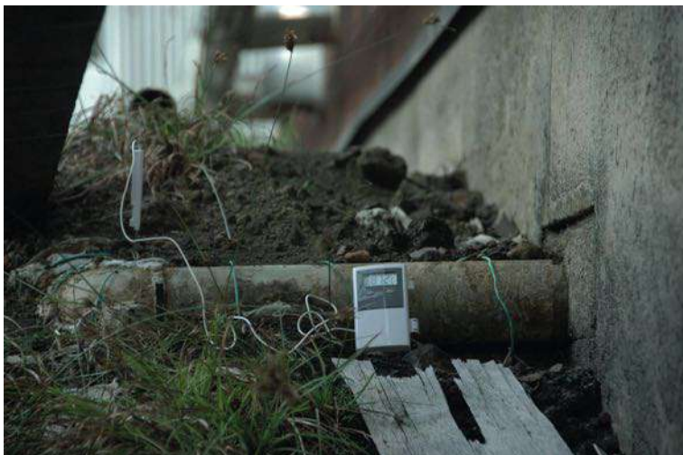
PHOTO 7 The geothermal steam inlet pipe extending from the buried heat storage tank into the saltworks.
