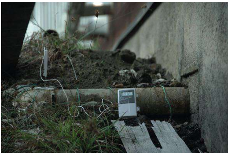
PHOTO 7 The geothermal steam inlet pipe extending from the buried heat storage tank into the saltworks.
