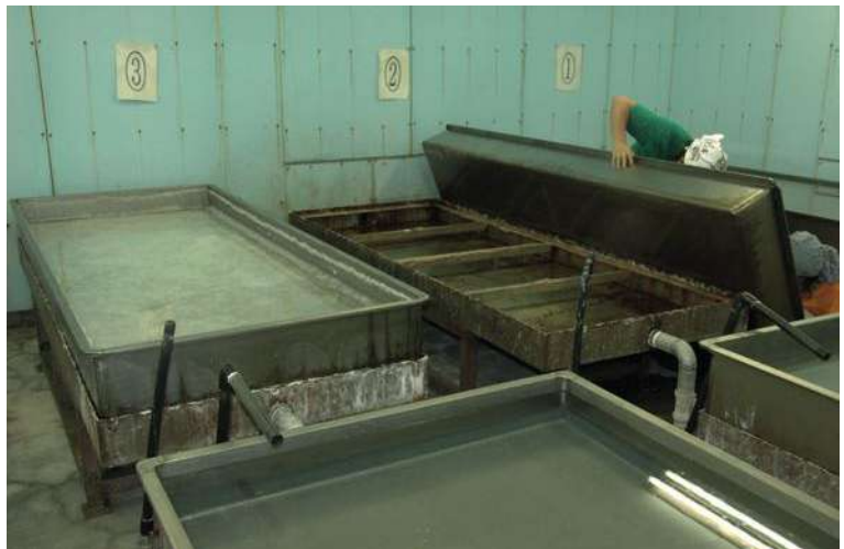
PHOTO 10 Stainless-steel geothermal steamers with titanium evaporating pans removed.
