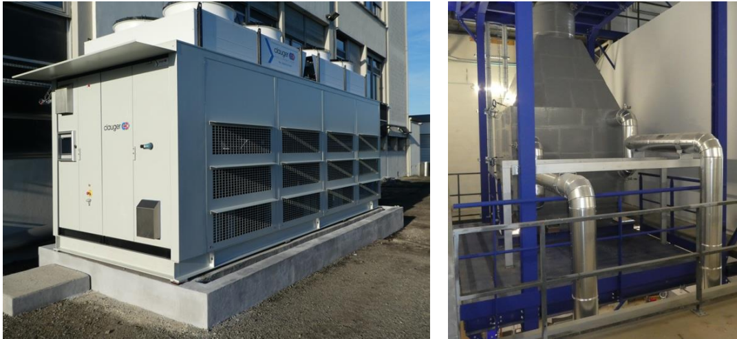
Figure 5: Cooling unit and heat exchanger
