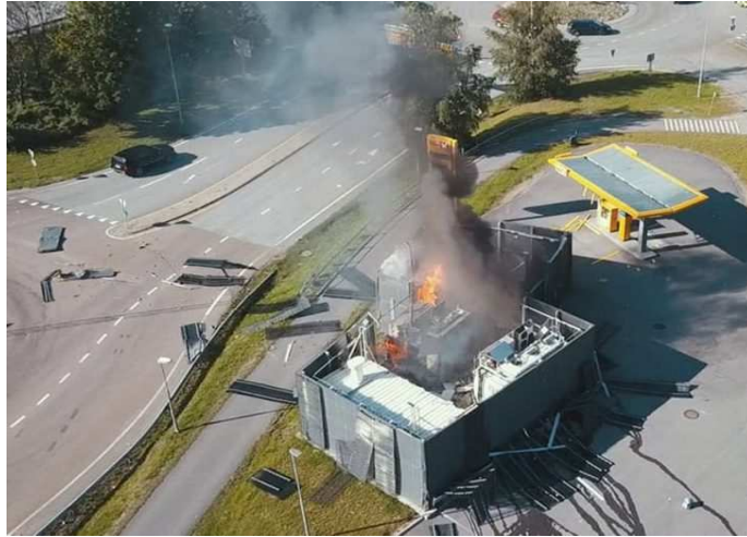
Fig. 3 Explosion at a hydrogen station (2019-Norway) [17]
