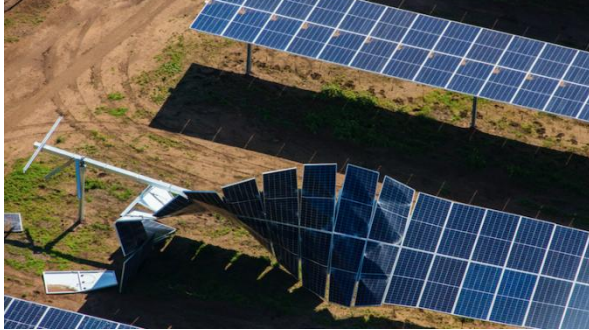
Figure 2. Single axis solar tracker facilities collapse (Source: www.pv-magazine-australia.com ).
