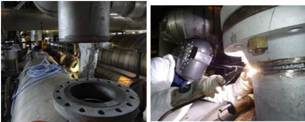
Figure 10. Installation of the flanges at the RV take-offs to hold the Type 2 perforated plates.
