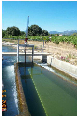
Figure 14. Example of sluice gate with a weir in an irrigation system.
