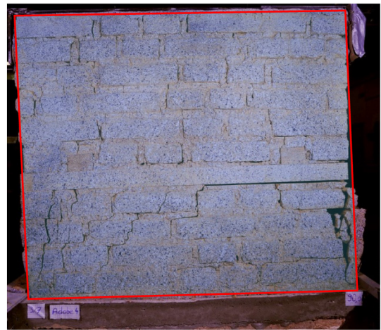
Fig. 14. Wall with timber band at 4560 s of loading at peak displacement towards left.
