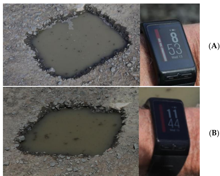
Figure 4. Low permeability demonstration of well compacted and slushed crushed stone base: (A) onset and (B) after a period. (A) Water level at start at 8:53. The sample hole was filled with water. Immediate seepage of moisture was visible at the surface (approximately 20–40 mm), but then becomes standing. (B) No significant reduction in the water level was visible over a period of three hours and was observed even over a period of 8 h.
