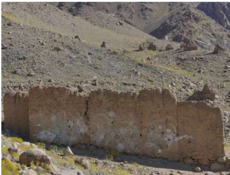
Fig. 43: View of the south wall of temple 1 showing the graffiti painted in 2013. ©MAFIL / R.S
