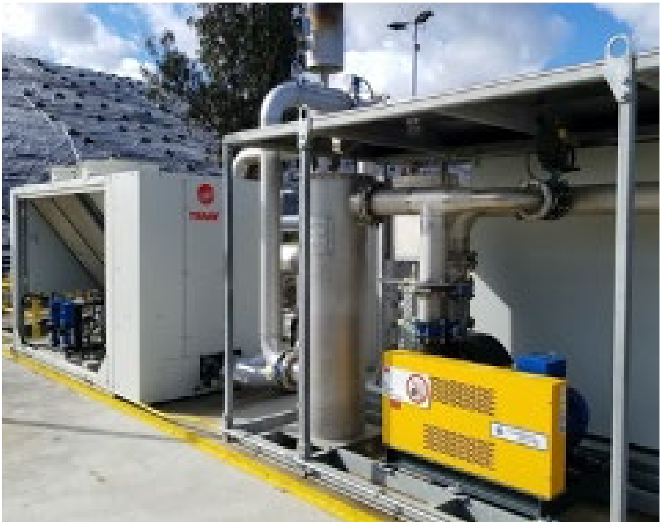
Figure 15. Copiulemu Landfill Gas Facility
