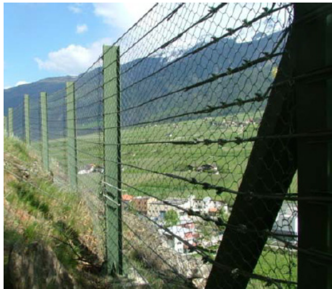
Figure 179: The Anas steel semi-flexible barrier type
