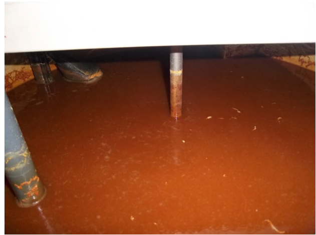
Fig. 2 An iron coprecipitation unit at the industrial scale. This technology is a well-known and well-accepted chemical process for the removal of metals and metalloids, including the removal of selenium and arsenic, and has been widely implemented in various industries; briefly, a ferric salt is added to the effluent, forming an amorphous iron oxyhydroxide precipitate; the trace elements are then adsorbed and trapped in the precipitate; the settled precipitate is then separated from the clarified effluent; with the technology of iron coprecipitation, metal concentration can be reduced to ppb levels
