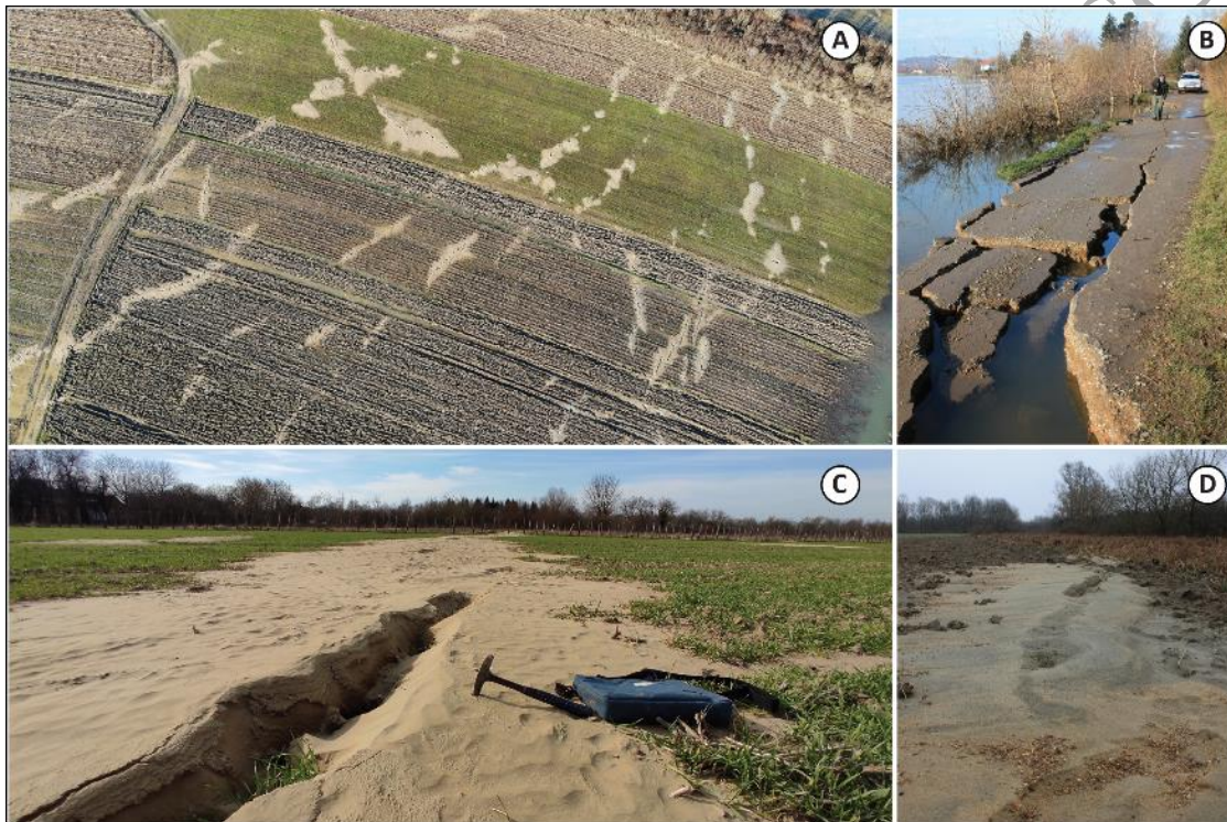
Figure 14: Examples of liquefaction following the Petrinja earthquake: (A) aerial view from drone at Letovanić (area 4 on Figure 15); (B) lateral spreading along Kupa river embankment at Letovanić (area 4 on Figure 15); (C) crack with sand ejecta in the alluvial plain of the Sava river; (d) sand and gravel ejecta of different provenance with presence of shells close to Kupa river.
