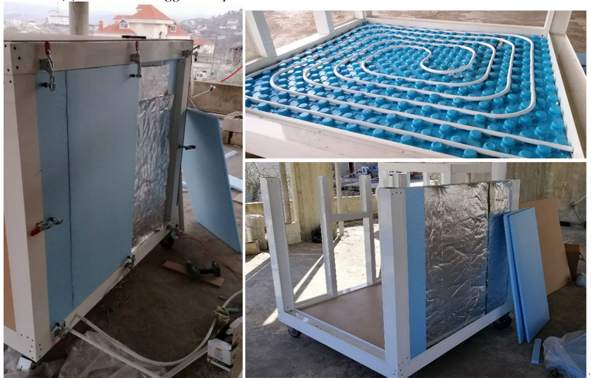
Figure 21. Real pictures showing different installed components in the implemented prototype.
