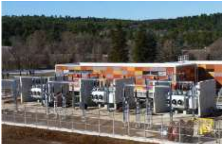
63kV / 15kV substation
