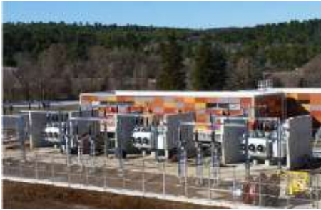
63kV / 15kV substation
