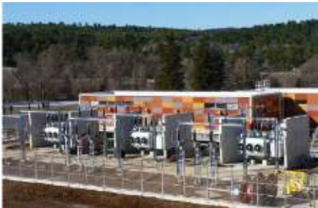
63kV / 15kV substation
