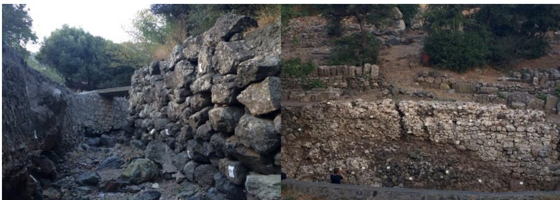
Fig. 4. Central Ravine. Intact section of Greek-phase boulder retaining walls (left); Intact section of Roman-phase concrete and limestone retaining walls (right). (© American Excavations Samothrace).
