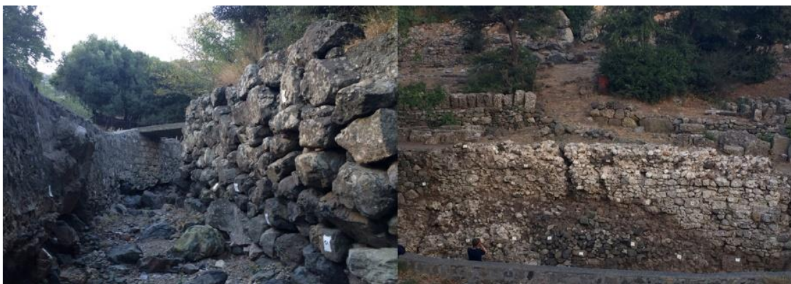
Fig. 4. Central Ravine. Intact section of Greek-phase boulder retaining walls (left); Intact section of Roman-phase concrete and limestone retaining walls (right). (© American Excavations Samothrace).
