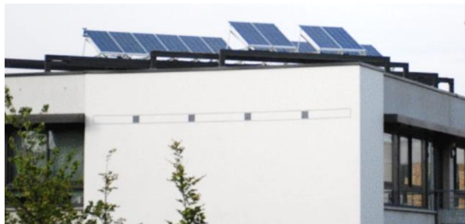
Figure 6. Photovoltaic installation of the Centre Pierre Guillaumat of UTC [17].
