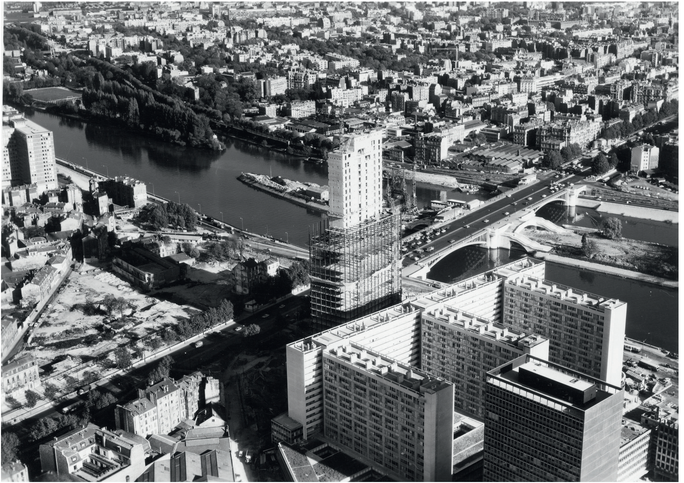
▲ Fig. 6. The Nobel tower block (PB31) under construction, photograph, ca. 1965 (© Archives départementales des Hauts-de-Seine).
