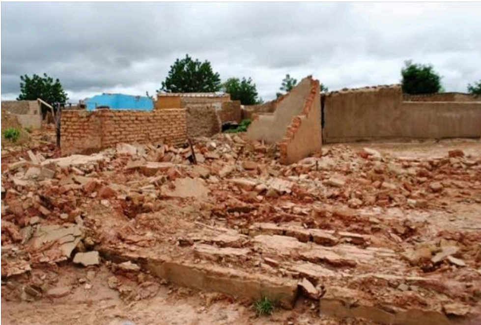
Picture 2: Collapsed house in the undeveloped area of Ouagadougou during the 2015 floods
