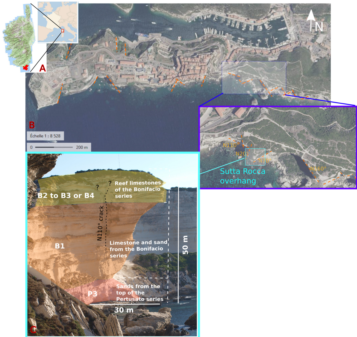
Figure 1. (a) Location map of the study area at the southern tip of Corsica island in the Mediterranean sea. (b) Detailed aerial view with the mapped faults of the Bonifacio formation (orange dashed lines). The coastal morphology is the result of erosion combined with tectonic accidents. Zoom-on the area of the Sutta-Rocca overhang. (Aerial photo Géoportail.) (c) Sedimentary sequence of the Sutta-Rocca overhang interpreted after Reynaud et al. (2013). From bottom to the top, unit P3: sands from the top of Pertusato series, unit B1: calcareous and sandy layers of the Bonifacio unit (B1) and units B2–B4: reefal calcareous rocks of Bonifacio series. The vertical N110° crack is marked by the dashed black line. The colour version of this figure is only available in the electronic edition.
