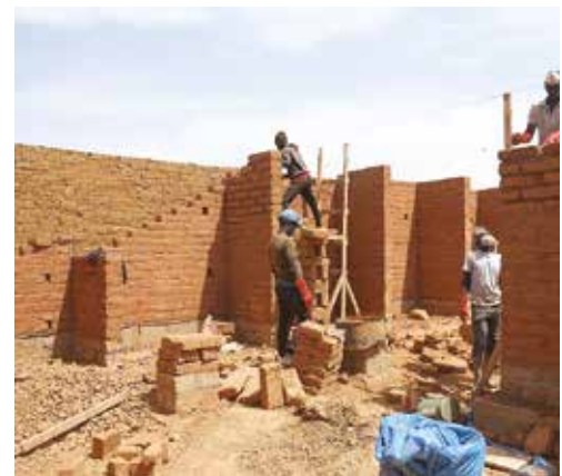
Building site of the first prototype of an improved granary in Matam
