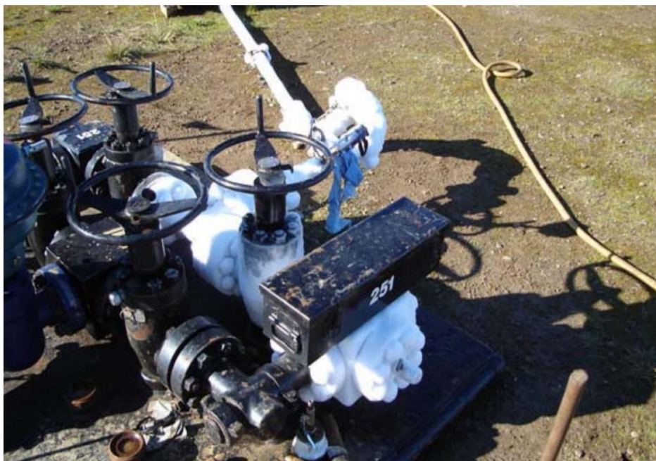
Figure 1. Ice formation from Joule–Thomson (JT) cooling on the exterior of the wellhead system of a CO 2 injection well where CO 2 vaporized from the liquid state to the gas state [35].
