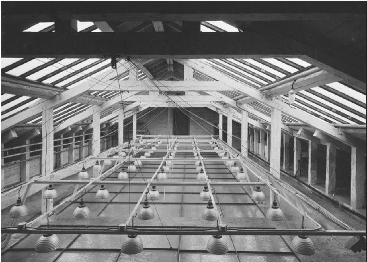
Figure 4 - Nationalmuseum, Stockholm. Lighting installation under the ceiling, second floor, painting room, 1931. Archive number 20/24. Ingenjörsbryån, SFV archive (The National Property Board). (© Nationalmuseum, Stockholm)
