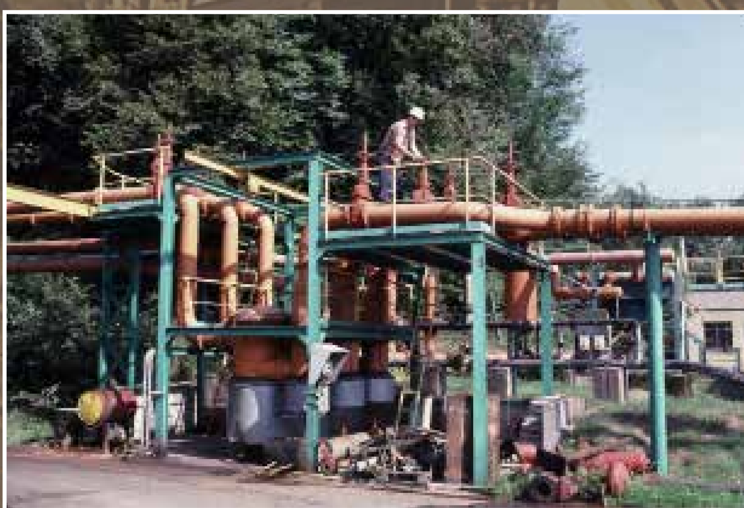
Station de captage de grisou sur le puits Peyerimhoff, Freyming-Merlebach, 1986 (B. Leidinger)
