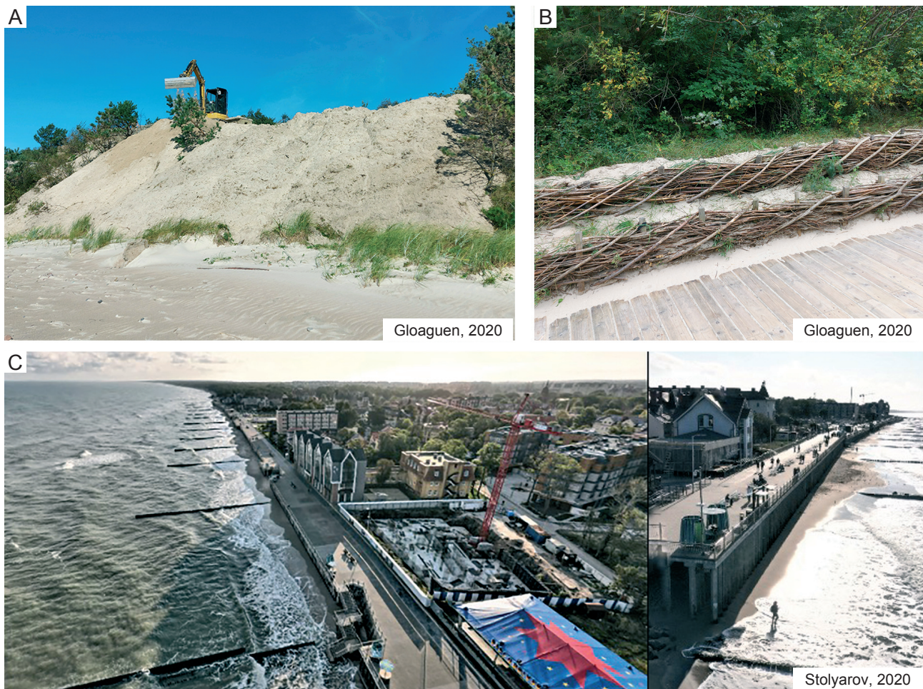
Fig. 7 Coastal protection measures. [A] Beach dune resurfacing and reinforcement works in the Lithuanian mainland coast. [B] Protection of the dune crest by natural materials with special fencing in Palanga. [C] Protective structures in the cities of the Sambian Peninsula, the beach is surmounted by several groynes and overhung by a seafront wall used as a promenade (with Google Street View)
