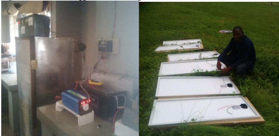
Figure 3: View of the Synchronization of the Constructed Egg Incubator and the Installed Solar System in Operation and View of the Solar Panels during Installation.
