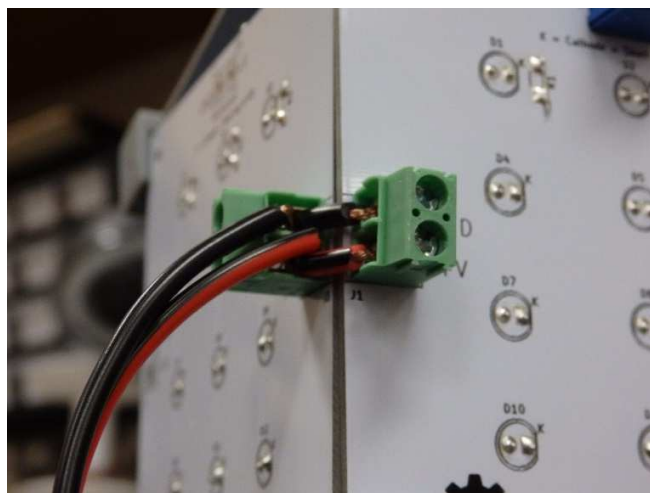
Figure 11. Two cables tapped into a terminal set for power flow from the supply
