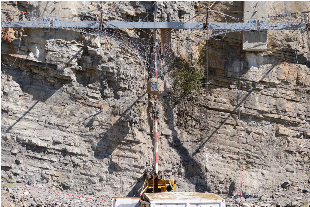
Figure 18: Front view of the quasi-static experiment on the rockfall barrier prototype (Courtesy of PN C2ROP).
