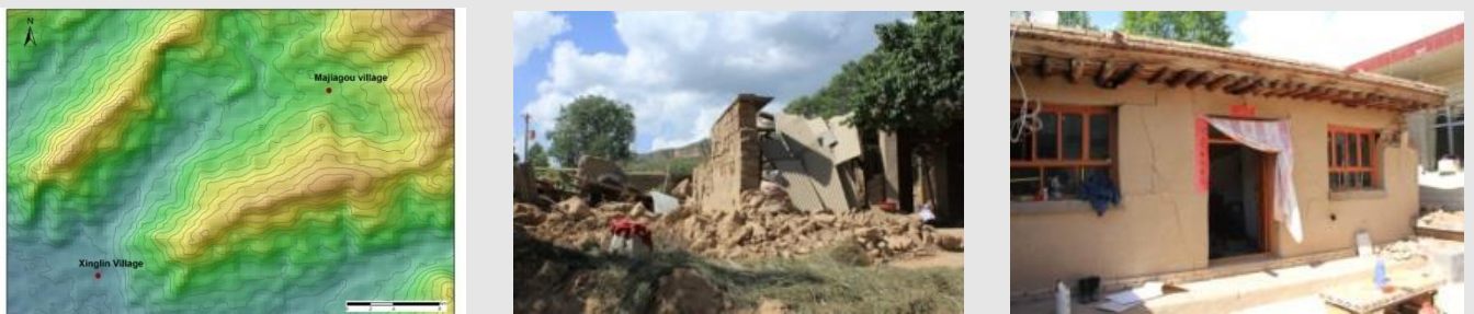
Fig. 5. The topography (left), seriously damaged houses in Majiagou Village (middle) and slightly damaged houses in Xinglin Village (right), Minxian Town, Gansu province
