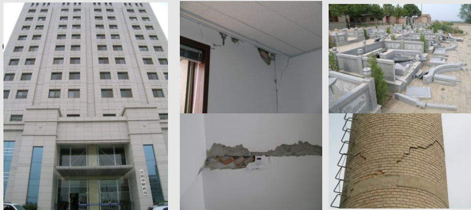
(a) A 12-stories reinforced concrete building on thick loess site. (b) Damaged walls in the building. (c) Damaged tombstones and chimney in the city.
