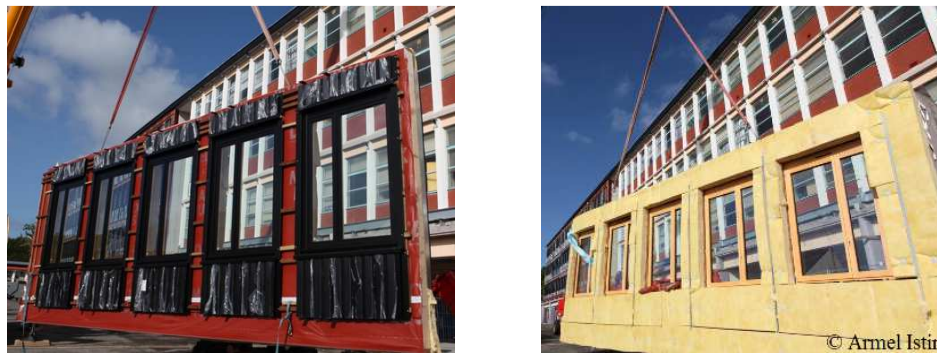
Figure 1: Views of the building before retrofit and the prefabricated ventilated façade element.
