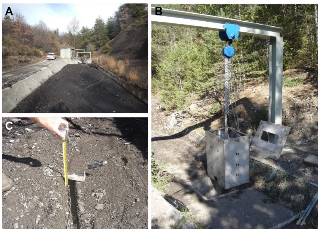
173 174 Figure 3. The 150 m 3 sediment trap (A), and the Reid (or Birkbeck) bedload slot sampler (B) used for 175 low and high frequency bedload monitoring of the Moulin Ravine, respectively; an example of scour 176 chain used for monitoring scour and fill processes in the Moulin channel is presented in panel C (©F. 177 Liébault).
