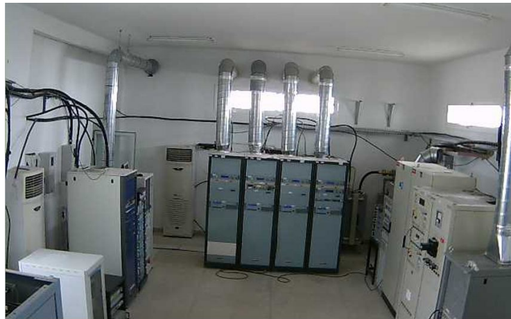
Fig 2: The equipment's TV and radio FM broadcast centers (S5)
