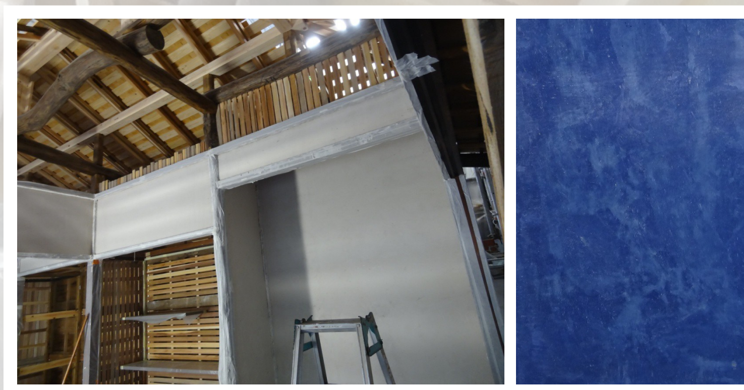
Left: East lodge being restored; Right: Blue paint test on plasterboard present on site.
